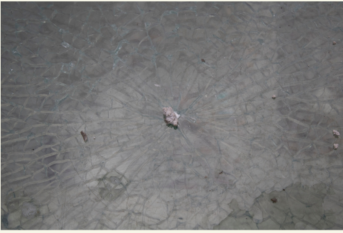
Plastic broken by bird shit
