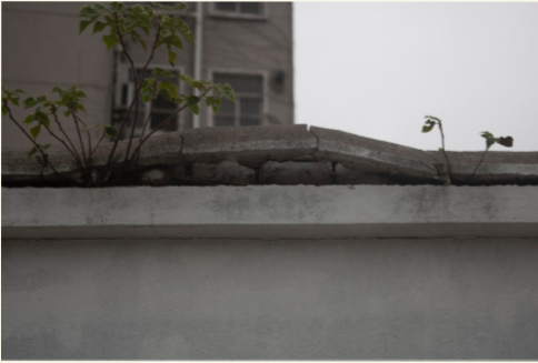
Wall broken by growing plant (maybe also by heat, rain and other things)
